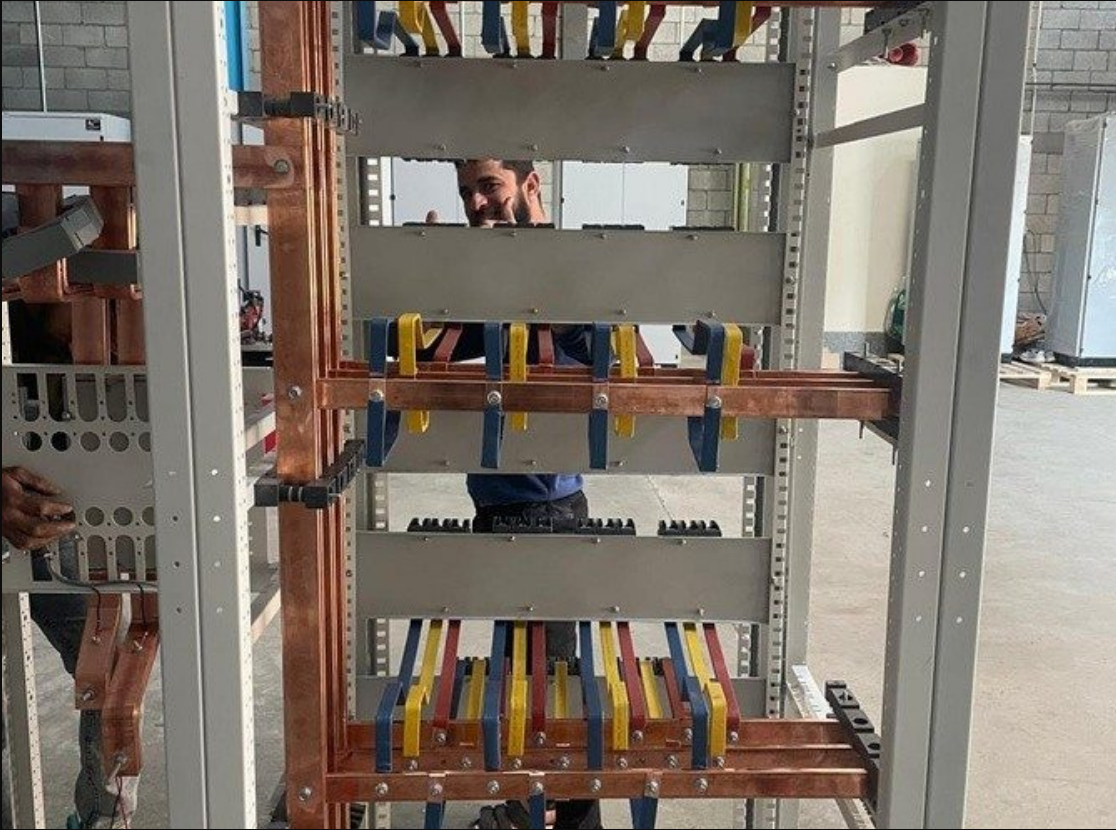
01 / Busbar and power assembly
